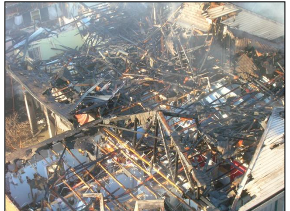
The roof of the medical building after the fire.
